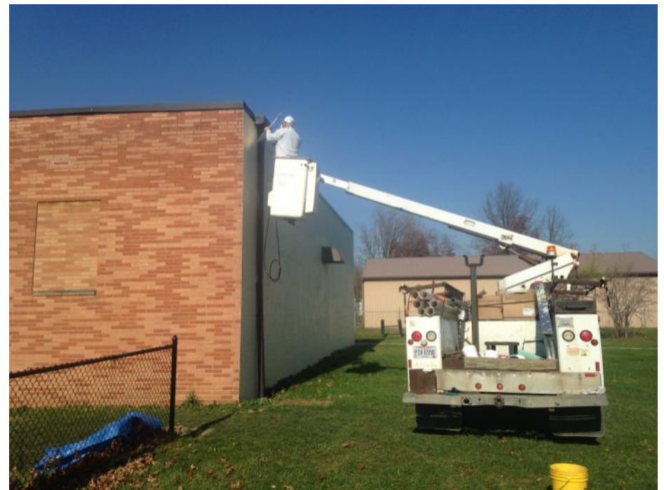
Br. Al Nugent paints the east wall of the Hall earlier this fall. PGK John Hricovec loaned the equipment for the day.
